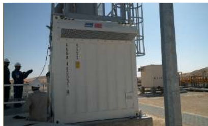
Power Generation Facility at Bisat Combustion Source Monitoring
